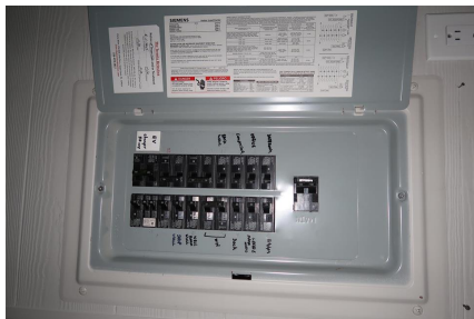
Sub panel cover on
