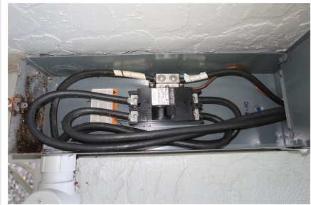
Main service disconnect cover off
