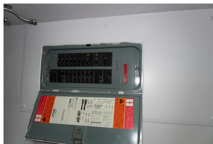
Sub panel cover on
