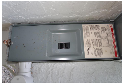
Main service disconnect cover on
