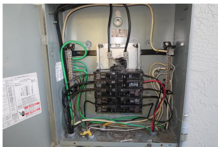
Sub panel cover off
