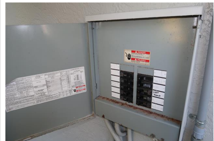
Sub panel cover on
